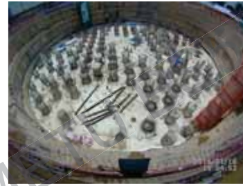
Figure 17 [2] : Raft Foundation The superstructure is supported by a four-meter-thick raft foundation slab and 137 cast-in-place board piles, each 2.2 meters in diameter and extending 60 meters in length. [3]
